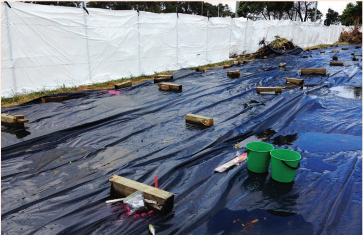
■ Figure 27. Temporary cover of contaminated soil.
