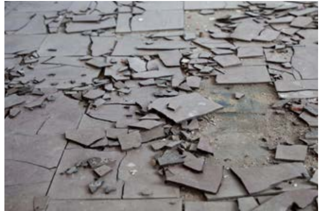
Figure 5. Tile and floor coverings containing asbestos in soil.
