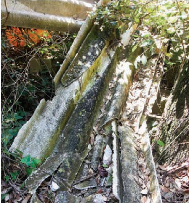
■ Asbestos-cement sheet fragments in soil from dumping or an old demolition.
